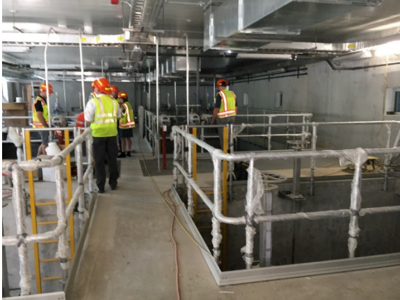
Dissolved air flotation treatment basins.
