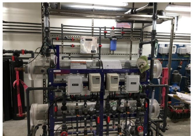
On-site hypochlorite generation facility.
