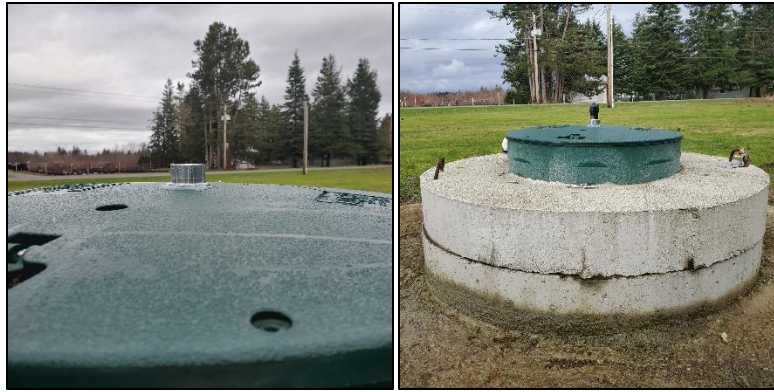
Figure 15: Top surface ground smooth with silicon and ½” watertight hub and nipple installed ready for the Ranger
