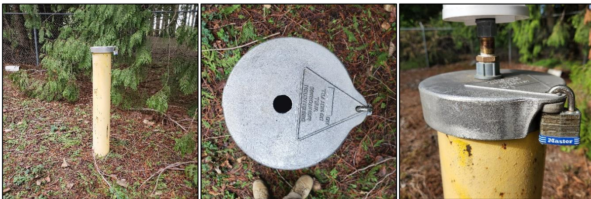
Figure 16: Monitoring Well 4” Aluminum cap with ½” hole, watertight hub and nipple installed with Ranger
