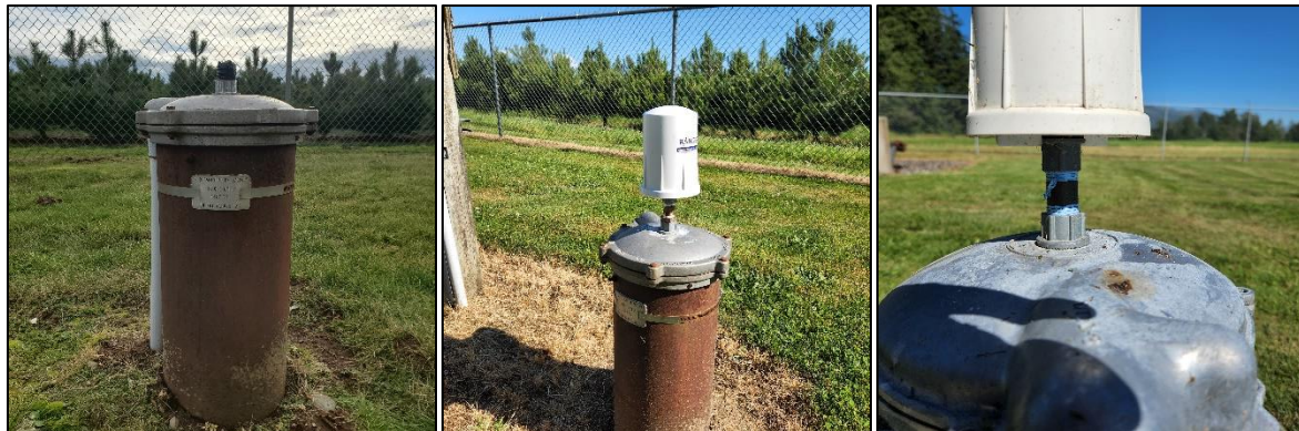
Figure 19: Wireless Telemetry Ranger Installed
